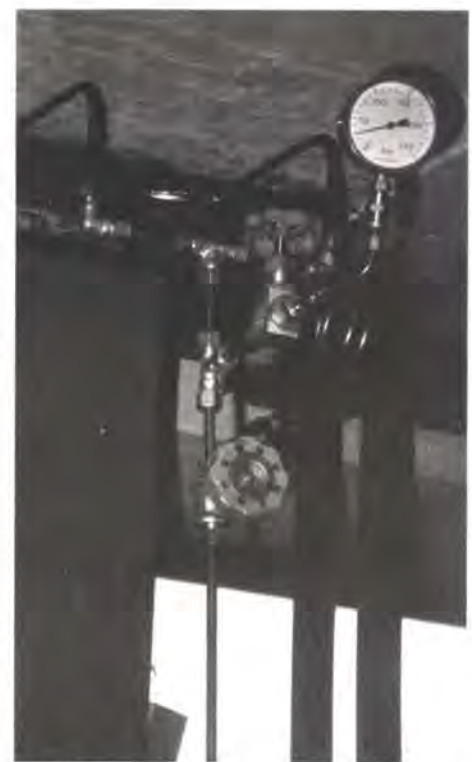
Fig. 11 Close-up of flat-jack arrangement at top of relieving stanchion (Photo: Poul Beckmann)
