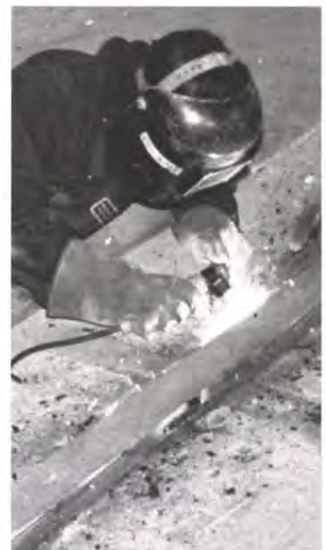
Fig. 8 Welding of strengthening plates to floor beams on Savoy Court (Photo: Frank Pyle)
