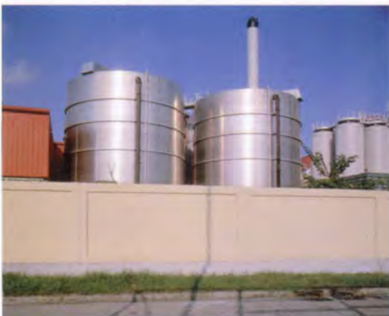
14. Water storage tanks.
