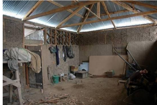
FigureA2-45 Internal view of large room with partially completed infill walls. Note the lack of bracing in any direction from the roof and apparently large distances between orthogonal walls. The system may be too flexible without enough support to the walls.
