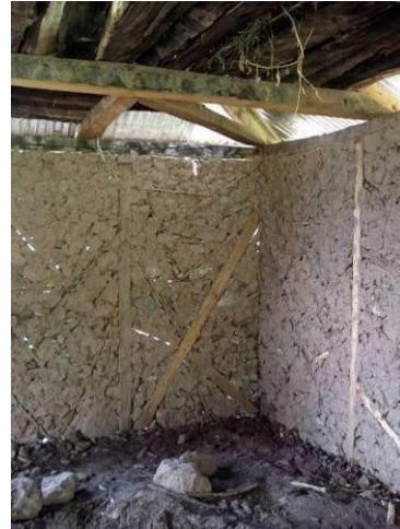
FigureA2-23 Internal view of completed wall. Note that the timber frame is not protected from getting wet as it is built straight in to the ground.
