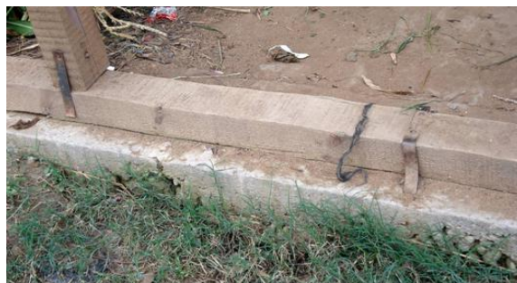
FigureA2-9 Timber ground beam (or sill beam) raised above the ground to protect the timber frame from rotting. Note attempted connection of the timber beam with the foundation. Damp proof course not provided.
