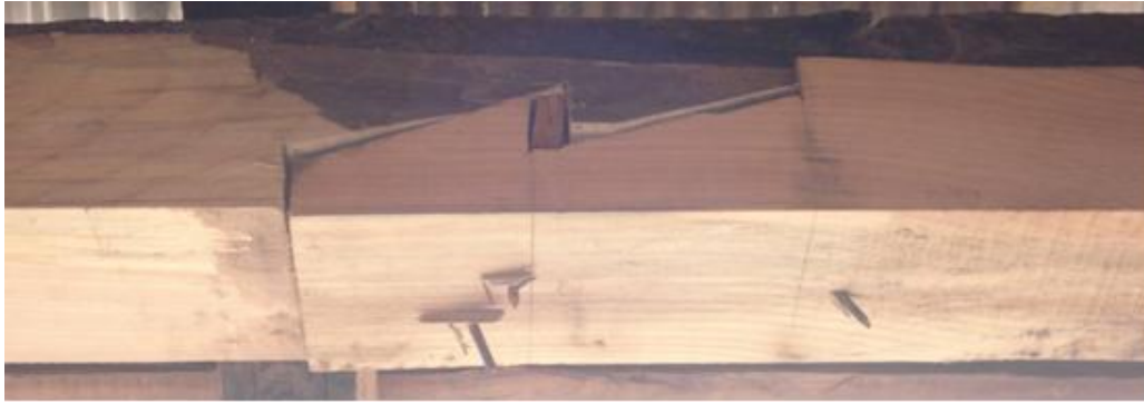
FigureA2-29 Poorly built scarf connection. The joint is a poor fit and the wooden peg that should pre-stress the joint appears loose. Note that the joint has been crudely reinforced with nails.
