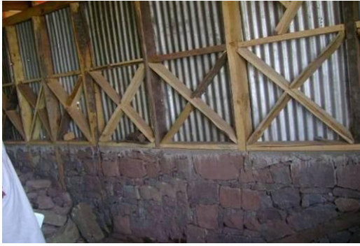
FigureA2-44 Mixed construction form. Dry stone wall with Dhajji timber frame on top but without traditional infill material. CGI sheets are used as cladding instead.
