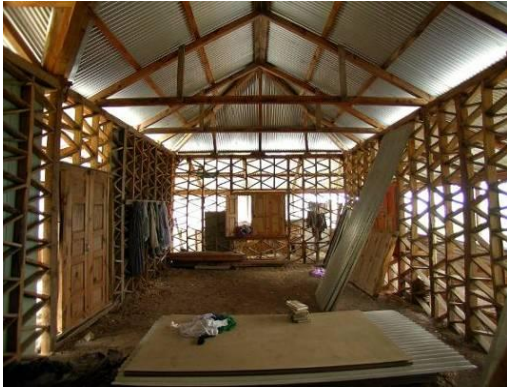
Figure A2-40 Inside view of a 1 storey house under construction. Note that the timber frame is in direct contact with the ground.
