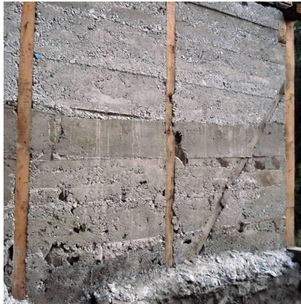
FigureA2-24 Timber, stone laid in concrete. This is not traditional Dhajji construction. There is a risk that the entire panel may fall out as a rigid object during an earthquake.
