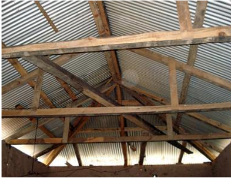
FigureA2-25 An internal view of a hipped roof. Apart from the CGI sheets there is no bracing to stiffen the roof structure
