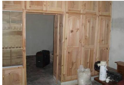
FigureA2-49 Full height built in wardrobe with reasonable thick solid timber back – possibly it acts in part as a timber shear wall but it is not a detail that the engineering solution should depend upon.
