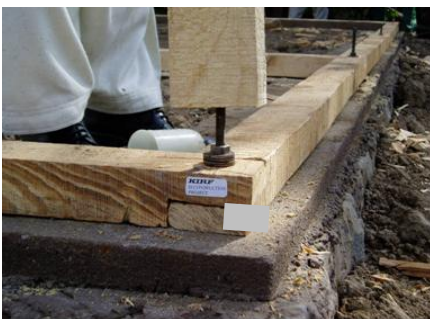
FigureA2-8 Bolting of plinth band with foundation. Note that a damp proof course has not been used
