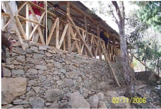
FigureA2-50 Dhajji frame built on a poor quality dry stone wall
