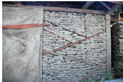
FigureA2-33 Large panel that appears to be poorly in contact with the timber frame. Lack of tight fit may result in the entire panel falling out-of-plane. Again note the layering of the infill due to local rock characteristics
