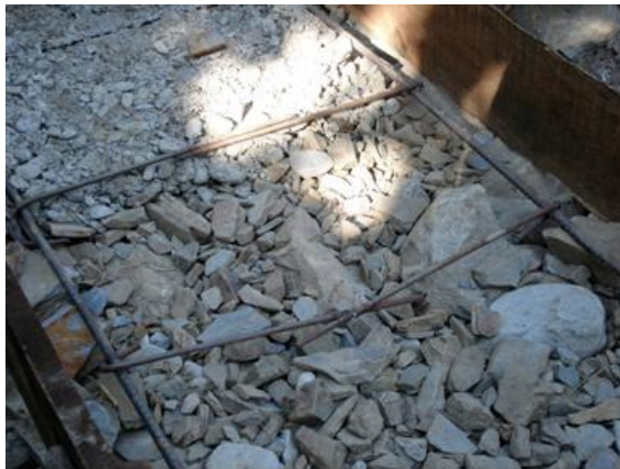
FigureA2-6 RC plinth band under construction (note poor splicing of stirrups)
