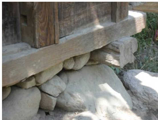
FigureA2-3 Foundation below plinth beam, note no connection between plinth wall and timber beam (existing building)
